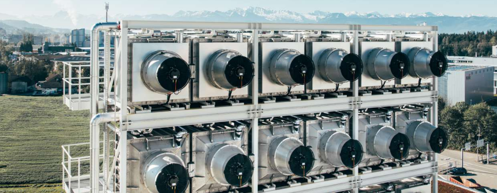
Fans for direct air capture at Climeworks' Orca plant
