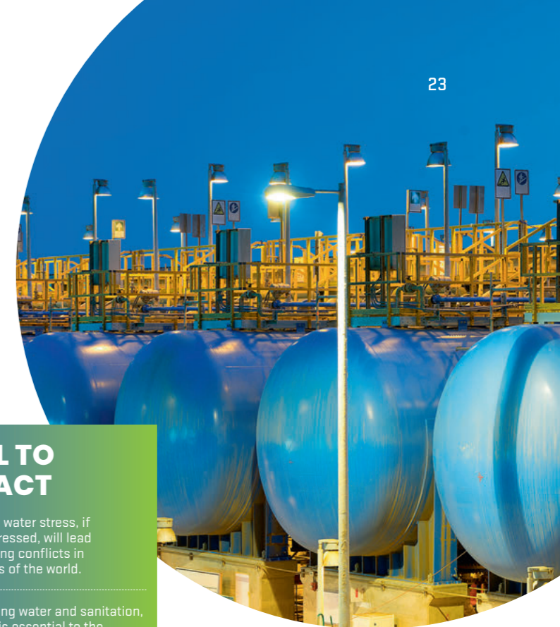
Reverse osmosis equipment in a desalination plant.
